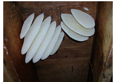
New wax combs between basement joists
